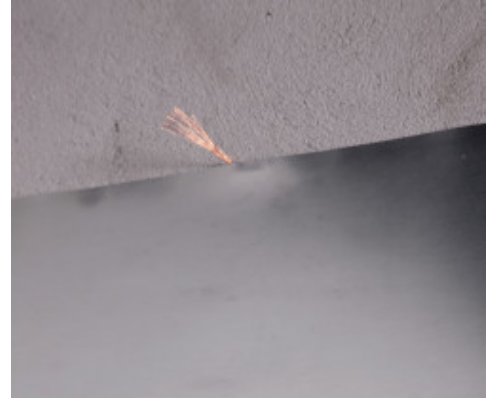
Electric wire previously connected to rebars
